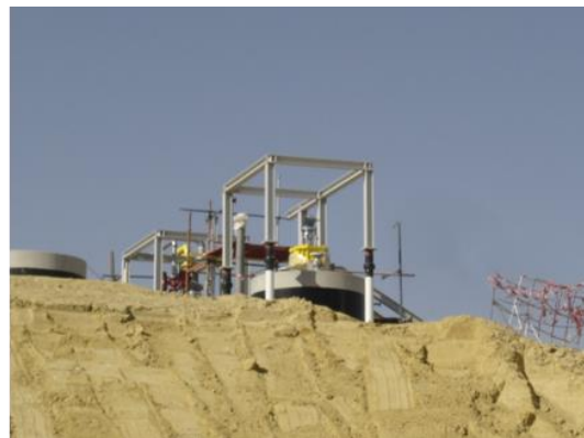
73BH installed on a “Cigar” Tank
